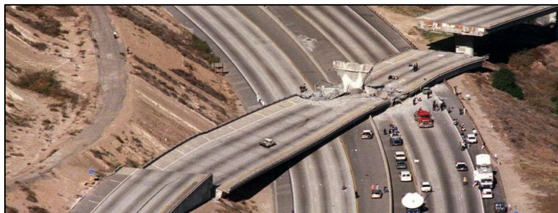
Figure 4: Overpass Failure in California after the 1994 Northridge Earthquake (6.7 Mw) - Source (University of California Los Angeles, n.d.)
